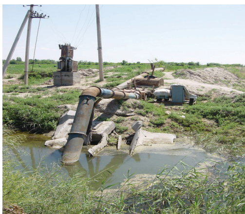
Deteriorated irrigation canal and water pump, Uzbekistan
