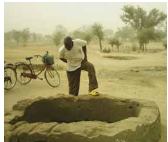
Poor maintenance of irrigation practices have resulted in the collapse of many irrigation systems.
