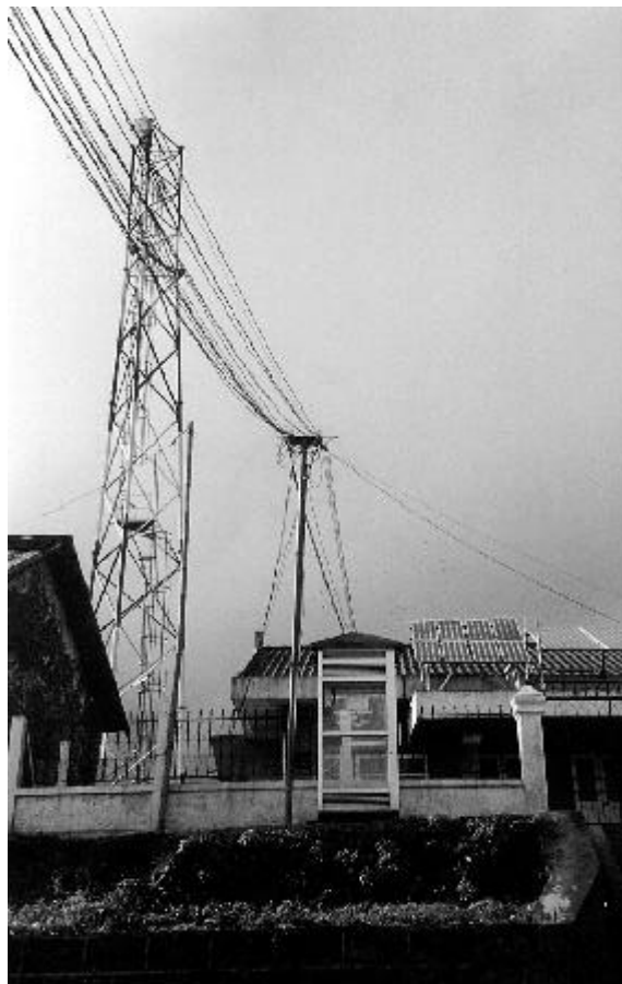
Telecommunication infrastructure in Laos.
